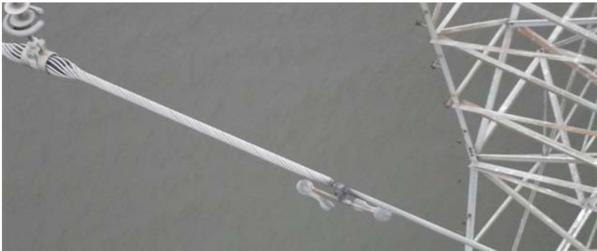
Attempted correction to fatigue at rod ends by placing dampers adjacent breakage locations unsuccessful
