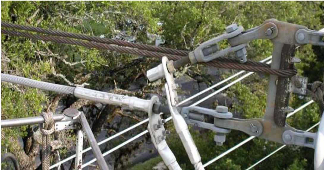
Typical catastrophic failure examples of single die compression deadends
