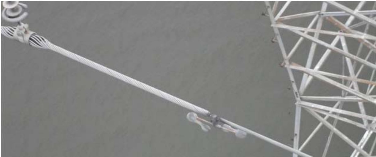
Attempted correction to fatigue at rod ends by placing dampers adjacent breakage locations unsuccessful
